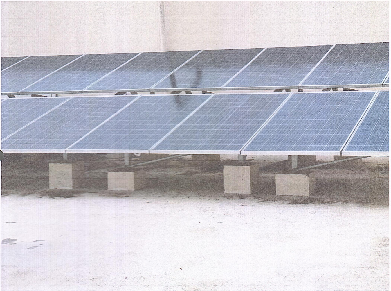
Solar rooftop installed at MAM College of Pharmacy
